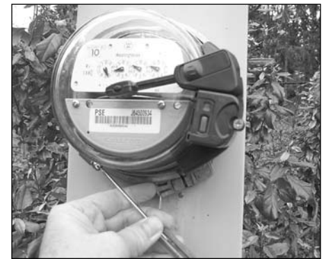
Outdoor device attached to PSE meter face.
